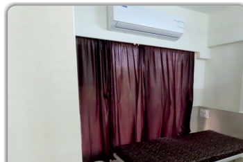
AC in Each Room
